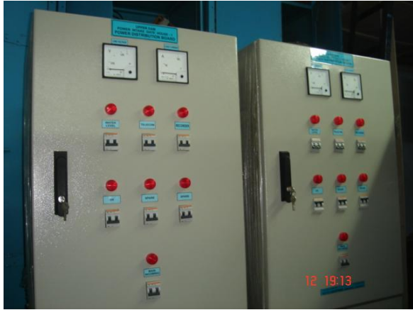
POWER DISTRIBUTION PANEL
