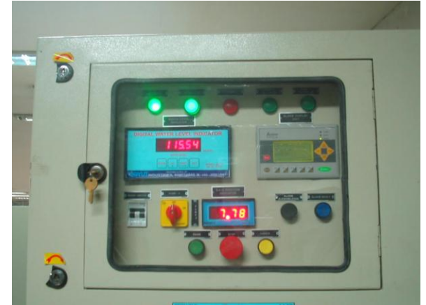
REMOTE PENSTOCK GATE OPERATION
